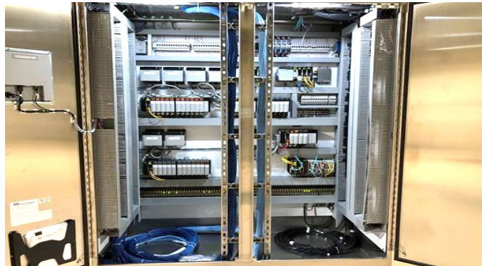
Typical SCADA Control Panel with Multiple Proprietary Components
