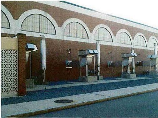
Air Compressor Building with Air Intake Ducts
