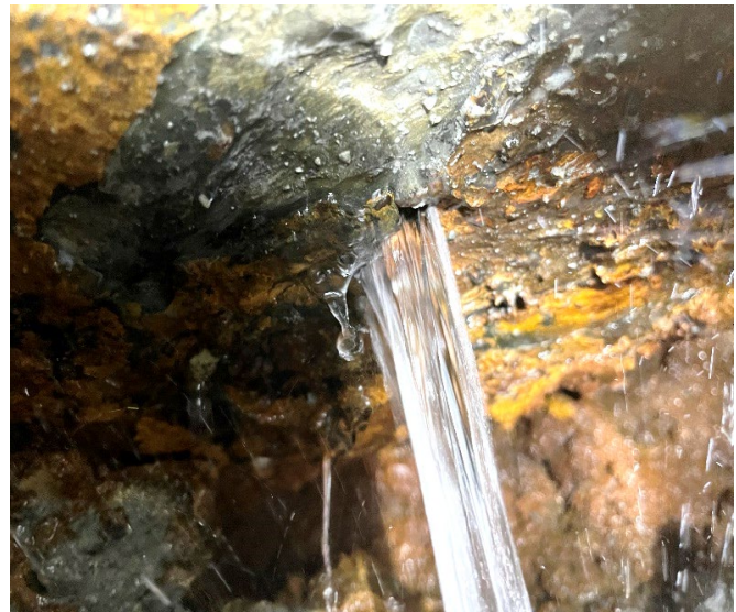
Figure 3. Leak Prior To Plug Installation
