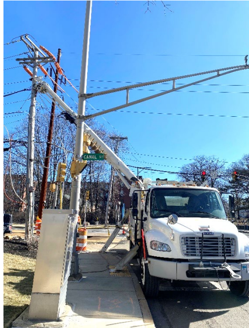
Figure 5 – Utility Pole Support
